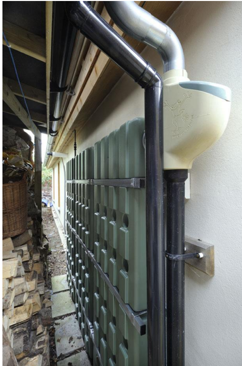
Rainwater is collected from the down pipe and used in the home
